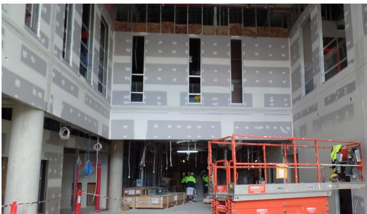
Above: Construction of the main Entry Foyer in the Acute Services Building.
